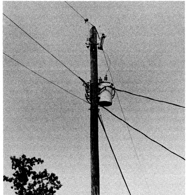
The fuse, which can be used to isolate individual lines, is located at the top of the pole. Note the large clamp on the top wire.
